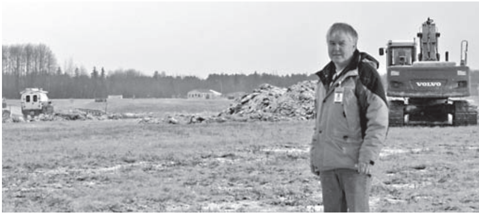
Joey Long stands where the new checkpoint to access 14 Wing Greenwood's airfield is under construction along Ad Astra Way.
