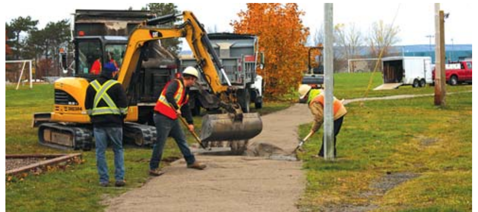
Crews work their way along, digging, leveling and gravelling new loops and pathways linking a network of trails around 14 Wing Greenwood's Residential Housing Units' neighbourhood and the Apple Bowl sports field. S. Keddy
