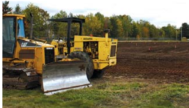
The Ivy Street ballfield will have new life come spring, following a three-way partnership to turn it into a quality – and needed – new soccer pitch. Levelling, irrigation and seeding the field has been a year-long effort by 14 Wing Greenwood, the Personnel Support Program and the Greenwood Soccer Club. S. Keddy
