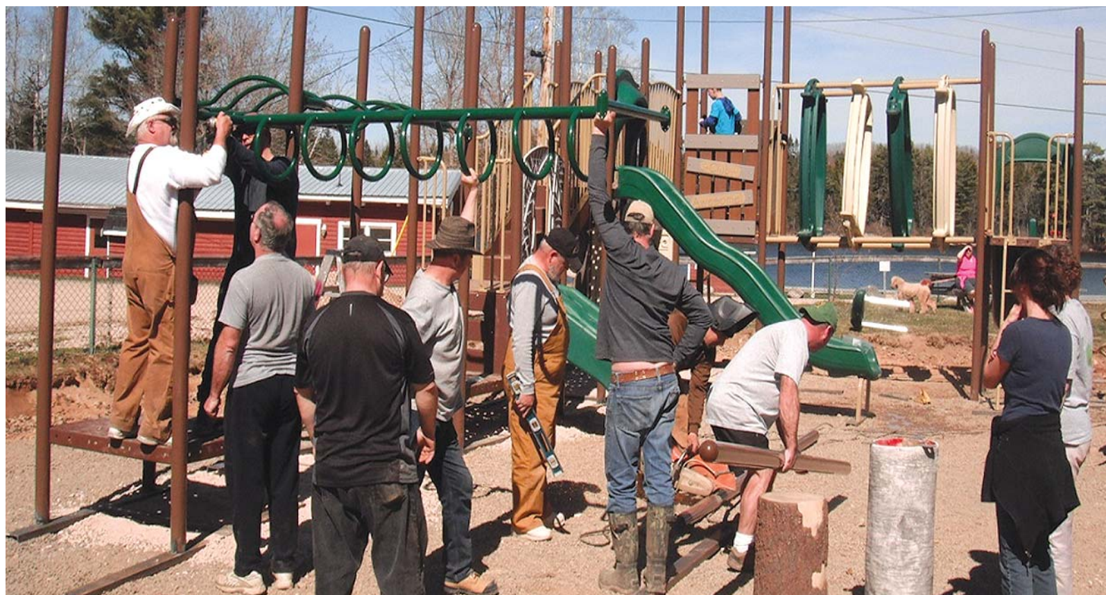
April 30 and May 1, a team effort tackled a new playground installation at the Lake Pleasant: Campground in Springfield. Campground staff and volunteers prepared the playground site and put together the new tree house-themed playground. Submitted
