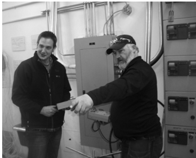
Department of National Defence energy manager Alex England, left, and Chris Malay from Advanced Energy Management discuss the installation of new damper actuators in the Annapolis Mess, one of several building automation system upgrades underway. Submitted
