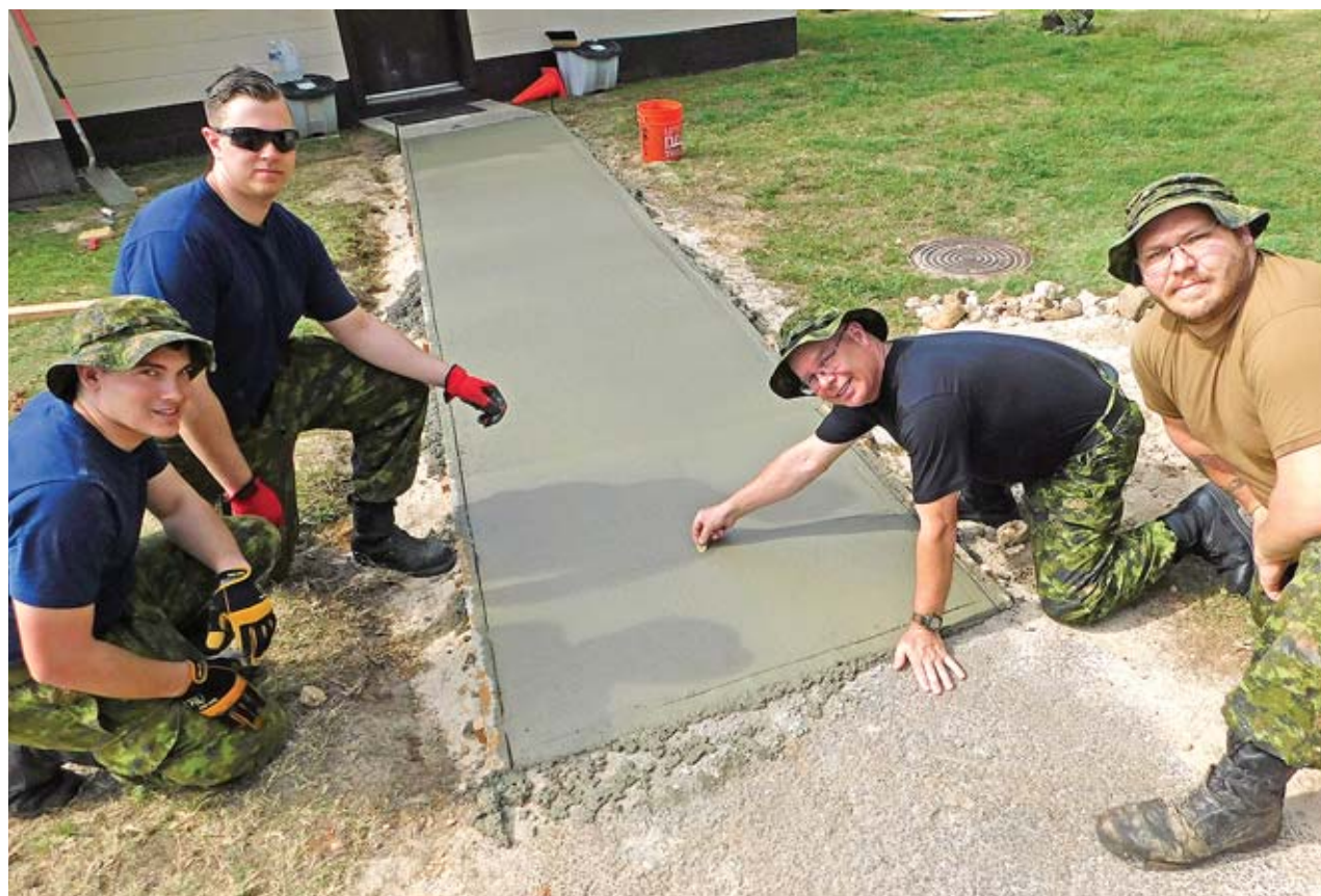
It wouldn't be a Canadian effort without adding a special touch: Petty Officer First Class Michael Dempsey, from 14 Mission Support Squadron's Construction Engineering Flight, placed a commemorative loonie in the concrete of one of over a dozen cement walkways poured while on deployed training at Bellows Air Force Station. Submitted
