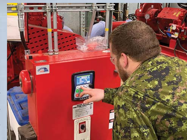
Electrical generating systems technician Aviator Rodden, confirming system parameters are within guidelines on #2 fire booster pump at Building 99 during a recent trouble call for a low coolant temperature alarm.
