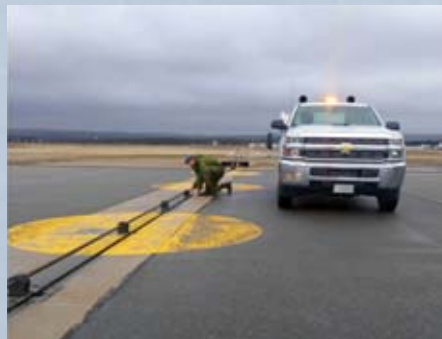
Corporal Luke Therrien, refrigeration and mechanical systems technician, checks the BAK-14 AAS support blocks to ensure they have not been damaged.
