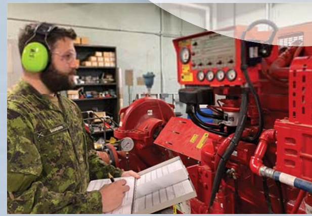
Private Saunders, electrical generating systems technician, confirms the analog gauges (engine data) are within spec during fire booster pump run-ups. EGS techs perform these tests weekly, paired with water, fuel and environmental technicians. These engine-driven pumps are a part of the wing's fire suppression system.
