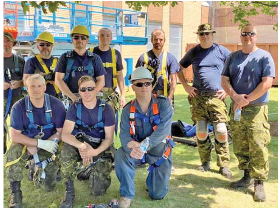
June 18, as most of us were thinking about shade and a cold drink, members of three Construction Engineering flights from Bridgewater (143 CEF, Pictou (144 CEF) and Gander(91 CEF) took to the heights on a joint repair operation of the 14 Wing Greenwood headquarters building. They crew was on site for over a week tackling the structure work.
