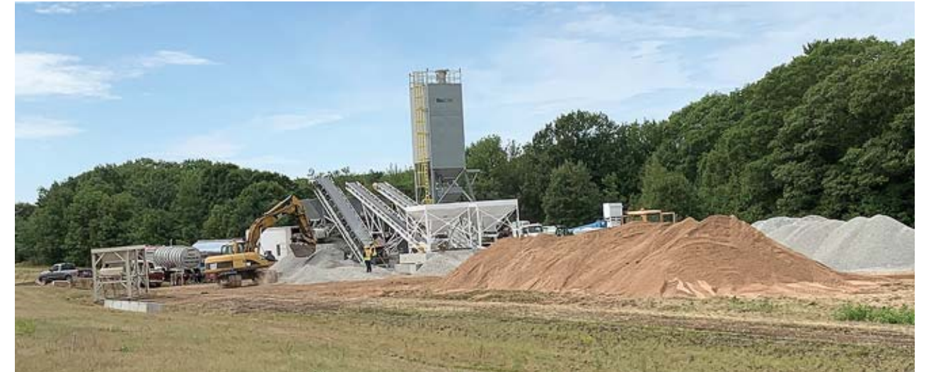
The $3 million job to replace Runway 1230’s paved button with concrete is underway: it’ll take 50 days of straight pouring to do the cement work alone.
