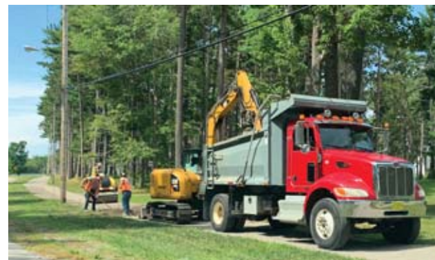
Repair crews spent time in August repairing 2019 sidewalk work along Kingswood Road. They’ve improved the drainage and rebuilt the sidewalk, after water pooled in the settled site last season.
