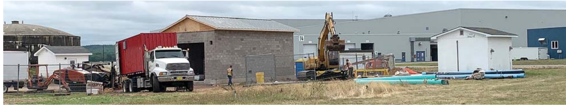
This new pump house on the operational side of the wing will be the final connection for Well 10 piping, coming under the airfield now. Once connected and tested later this fall, it means potable water on the ops side – the first since 2010.
