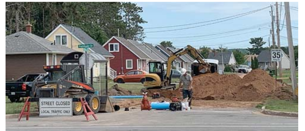
In the first phase of a five-year project, this summer’s work under 1st and 2nd Crescents will replace all the old iron main and lateral water lines to Residential Housing Units.
