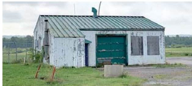
Four 1950s- and 1960s-era buildings, including this one, in 14 Wing's Explosives Ordnance Disposal area that used to house missiles, bombs and torpedoes will soon be demolished.
