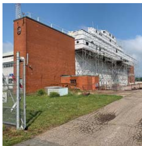
Work on 9 Hangar continues, but 14 Operations Support Squadron should have the fully renovated building in its hands later this fall.
