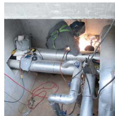
This is a steam vault, where the new connection to feed Building 172 is being installed.
