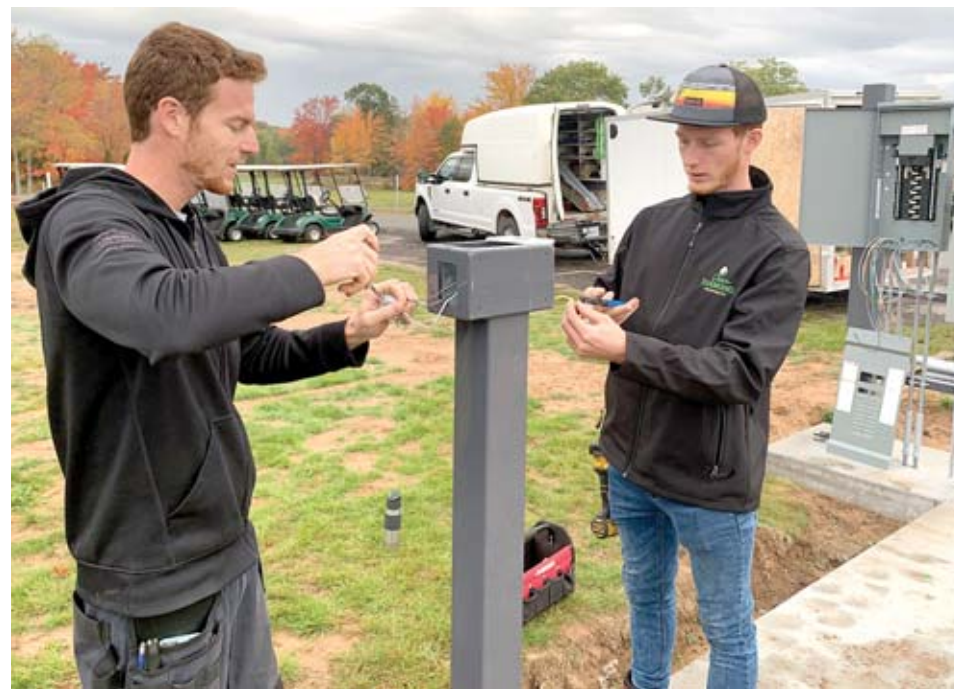
Doyle Barkman, left, and Neil Barkman of Terrawatt Electric install the components of the electric charging stations for the Greenwood Golf Club's transition to an all-electric golf cart fleet for the spring of 2022. S. White
