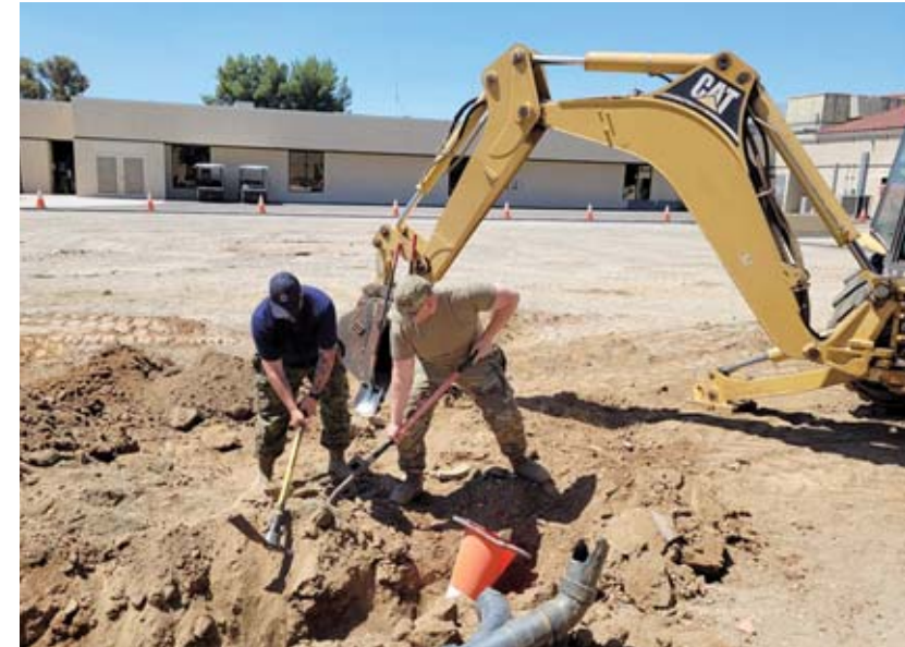
Corporal Patey from 91 CEF Gander working with Staff Sergeant Kevin Au, a Water and Fuels System Maintenance (WFSM) technician assigned to the Civil Engineering Squadron (CES), 107th Attack Wing, NY Air National Guard, Niagara Falls Air Reserve Station.
