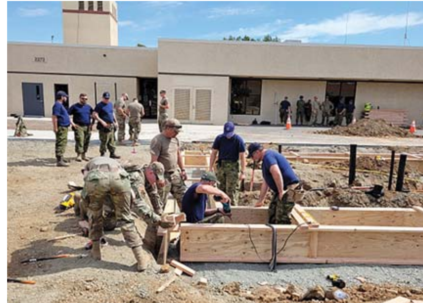
Several members of 14 CES and 107th Civil Engineer Squadron working together on the footings for a restroom area at March Air Reserve Base CA.
